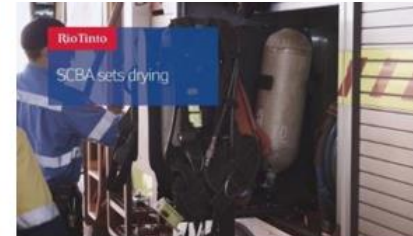
SCBA lockers let open to allow for drying
